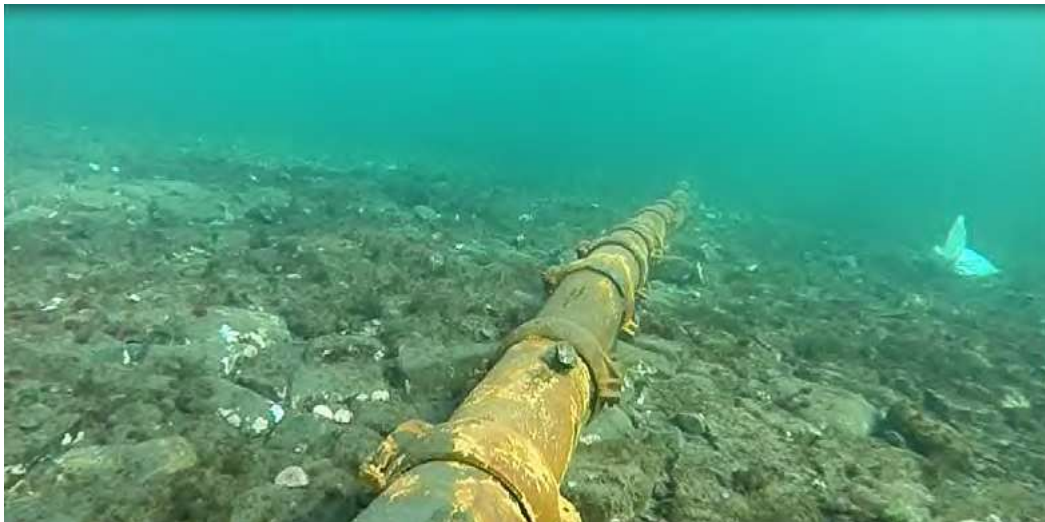
Cast Iron Sells for Cable Protection (Broad Cove)
