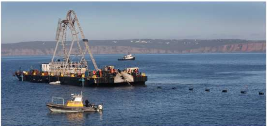
Floating part of the cable in the 1 st landing point (Broad Cove)
