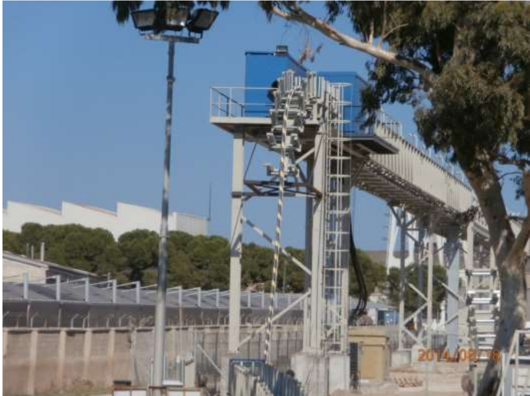
Dedicated loading line between the factory storage tanks and the port
